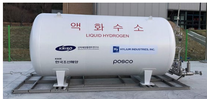
Figure 17. A cryogenic tank for the storage of liquid hydrogen.
